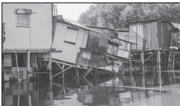
脆弱且危險的建築結構 Weak and Dangerous Structures
